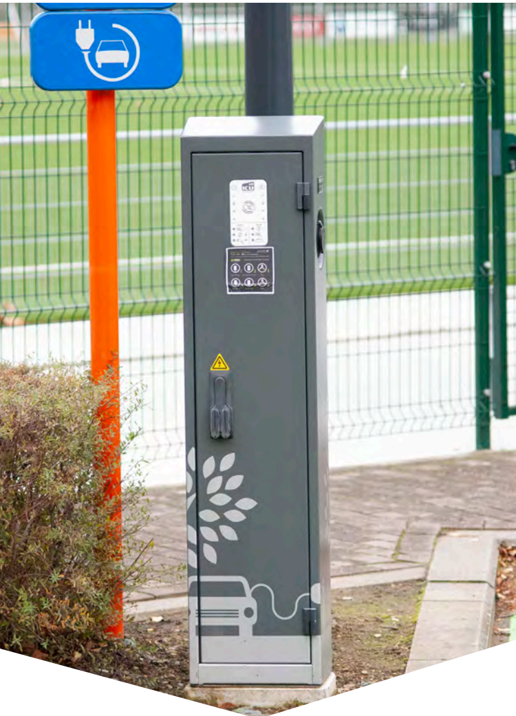
foto: Laadpaal parking Colomba
